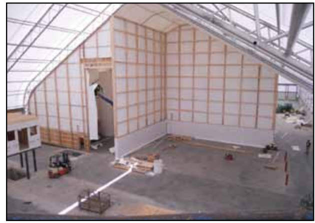
TAKING SHAPE. The new Ashley, Mich., facility is being assembled, and already some warehousing of raw materials is taking place.
